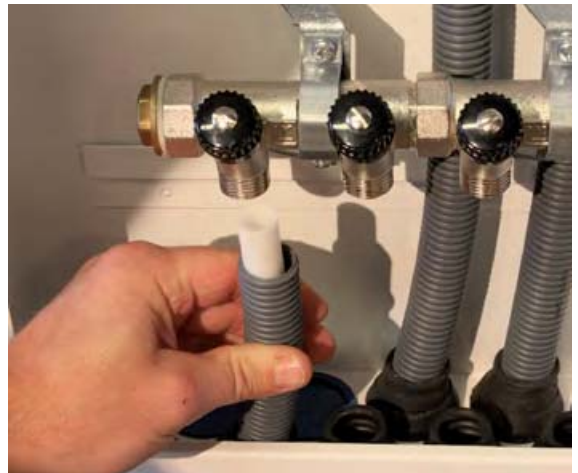
9. Pipe in conduit is then drawn upwards into the cabinet pipe inlet and is cut/deburred.
